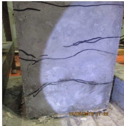
Cracks at the Hinge
